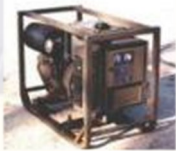
2kW Military Tactical Generator (MTG)
