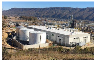
Natural Gas Steam Facility
