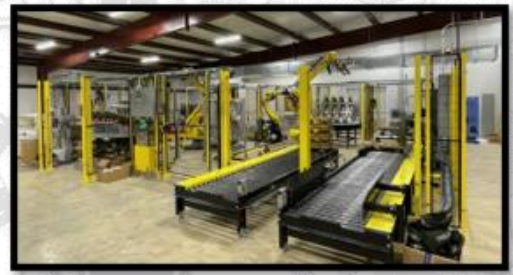
LAP Automated Receiving Inspection at Camden, AR
